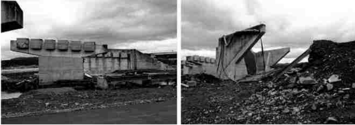
Figure 1-2: Deck Sections Displaced from the Piers and Abutments (left); Severe Scour behind Abutment (right) (2011 Great East Japanese Earthquake and Tōhoku Tsunami, Robertson, with permission from ASCE)
