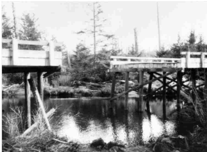
Figure 6-3: Joe Creek Bridge Damage from 1964 Alaskan Earthquake and Subsequent Tsunami (reprinted from TsuInfo Alert, [February, 2014])
