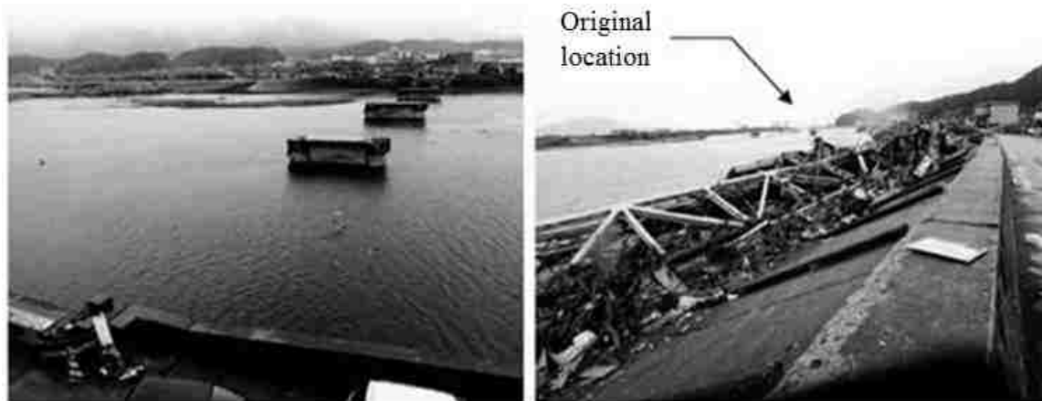
Figure 1-4: Steel-Truss Road Bridge Swept up to 800m Inland from its Original Location due to the 2011 Great East Japanese Earthquake and Tōhoku Tsunami (2011) (Robertson, with permission from ASCE)
